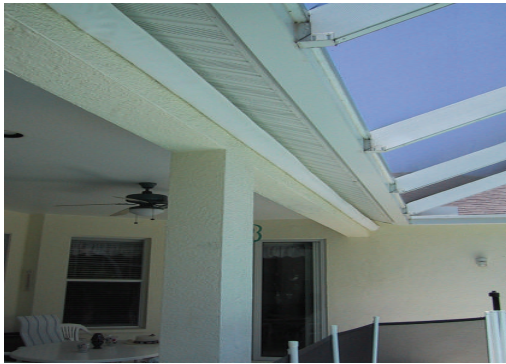
Hurricane screen mounted and rolled under eave, barely noticeable.
